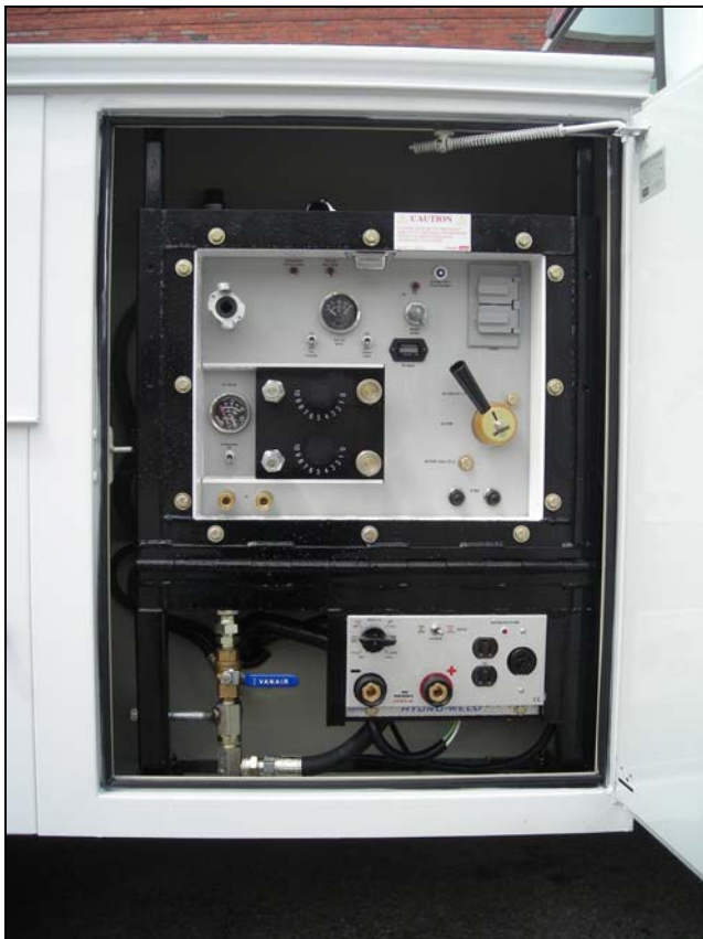
2042P Control Panel
